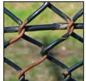
Standard extruded PVC coated wire with damaged PVC coating and red rust to exposed core wire
